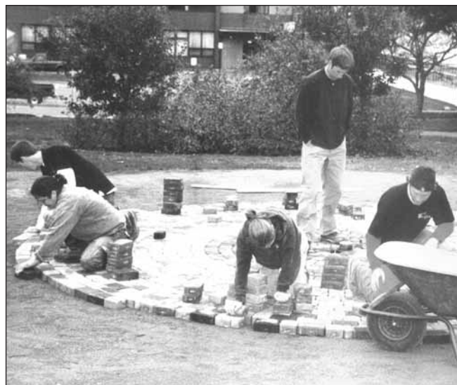
NSAC students participating in the construction of the labyrinth pattern in the Amphitheatre floor.
